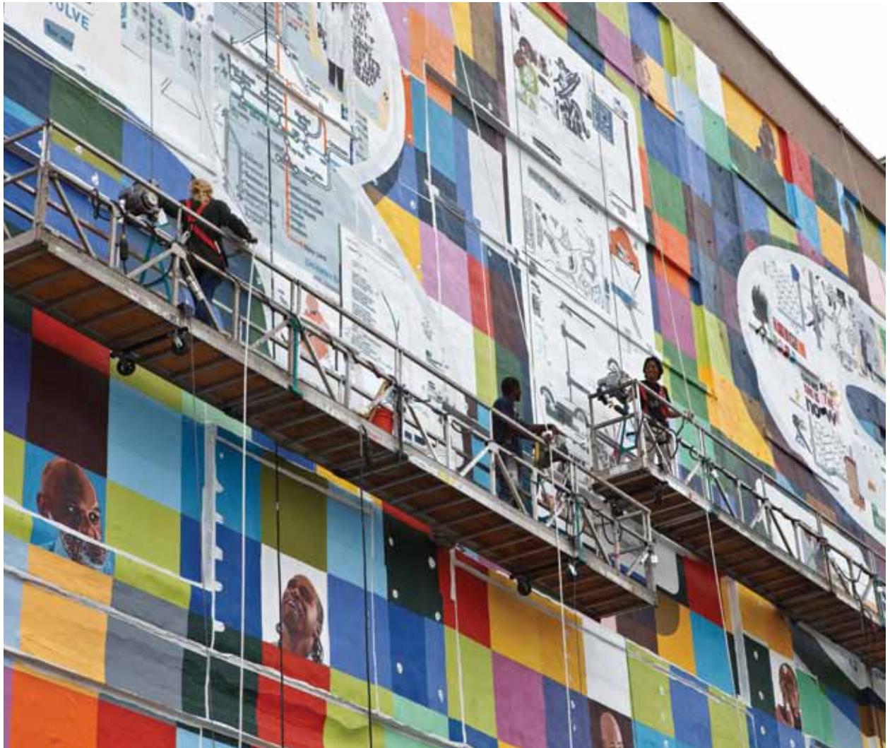
The North Philadelphia Beacon Project in progress, August 23, 2013. Photo by Steve Weinik.
